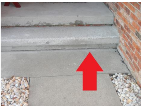
Settled concrete walkway.
