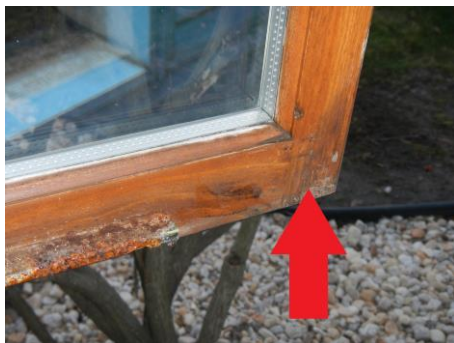
Damaged dining room windows.
