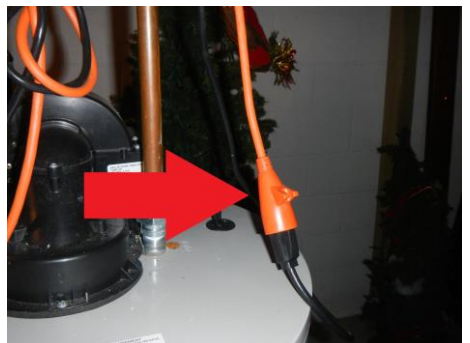
Missing outlet at water heater.
