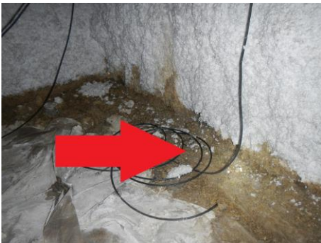
Water intrusion in rear crawl space.
