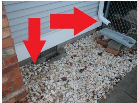
Improper grade and downspout.
