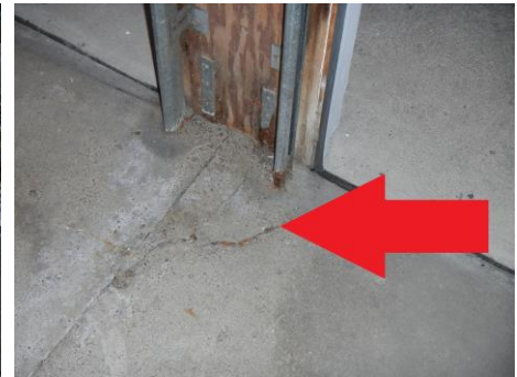
Damaged garage floor.
